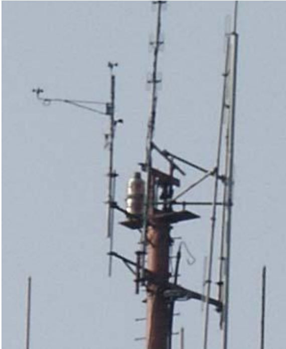
Figure 2 - Instrumentation at top of Yankee Network Tower – note the anemometers on the left (horizontal boom and at the top of the left-hand vertical tube).
