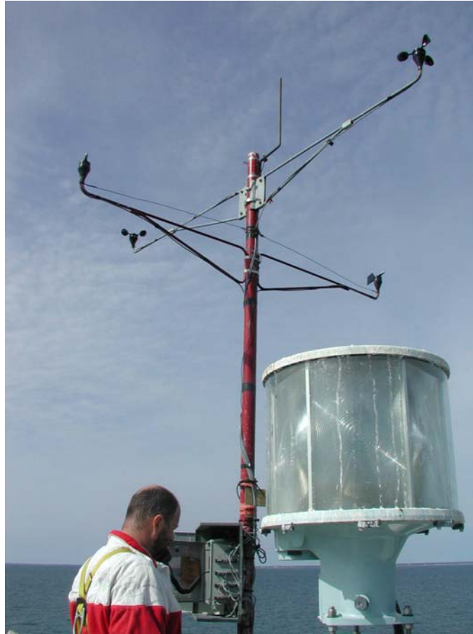
Figure 2 - Anemometry mast and data collection equipment at Bishop & Clerks
