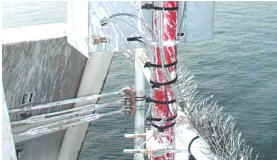
Figure 3 - Railing stiffener connecting PV bracket to rail
