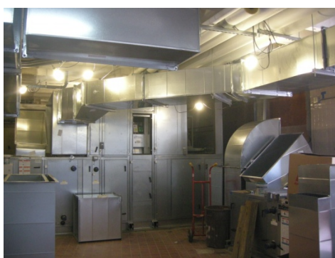
The new heating ventilation and cooling system in the pilot plant in the space formally occupied by the smoke house.
