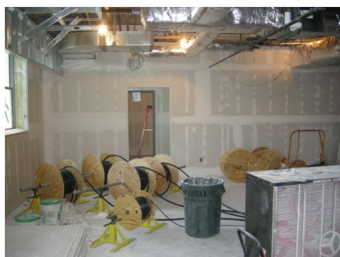
One of the new labs in the Fergus Clydesdale Foods for Health and Wellness Center. The wires are for the electrical upgrade for the entire building.
