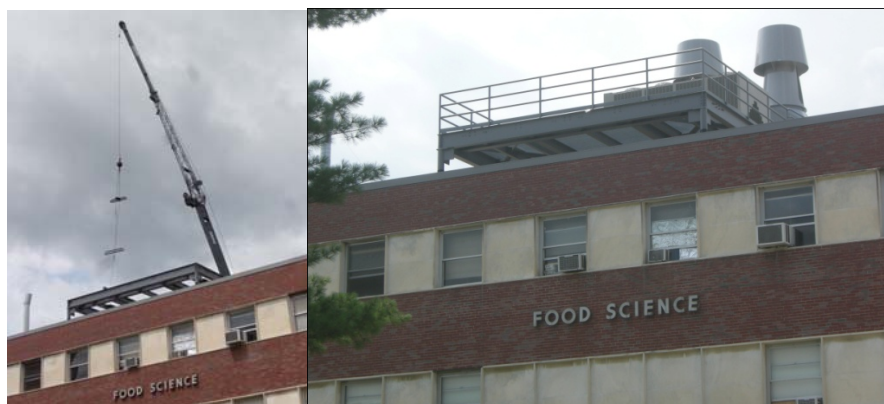
Placement of the heating, ventilation and fume hood on the top of Chenoweth.
